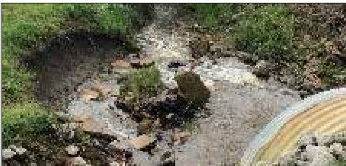
Figure 8. Pre-treatment bank conditions at a farm culvert.
