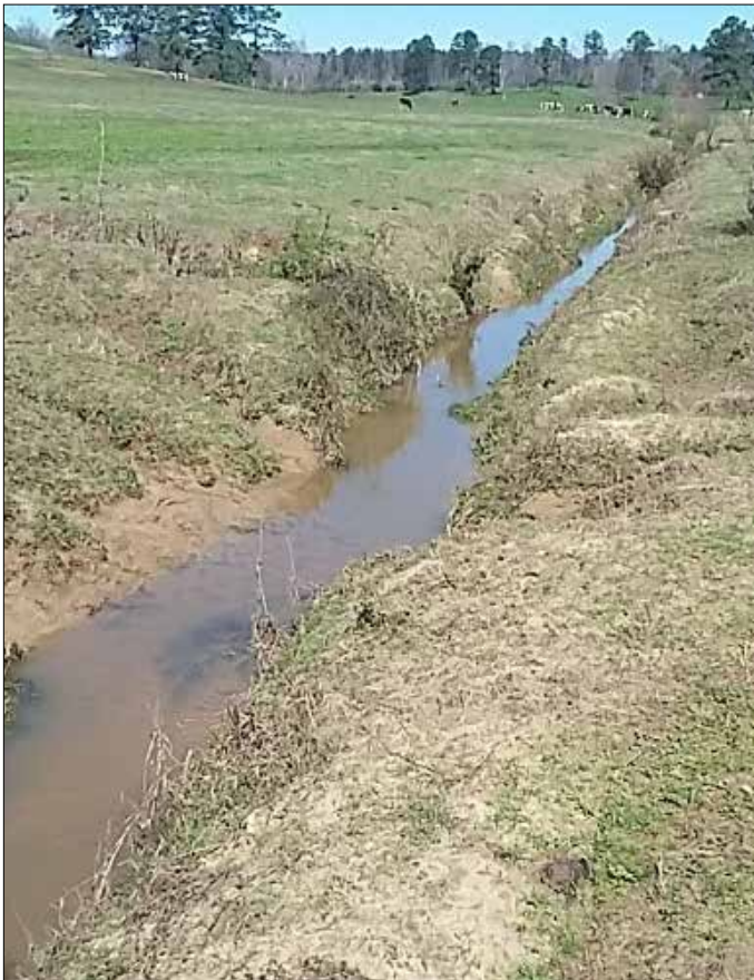
Figure 2. Stream conditions prior to implementation of best management practices.
